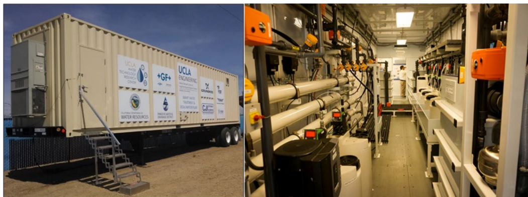
Figure 7. (Left) Mobile two-stage RO plant trailer, and (right) inside view of the plant.
